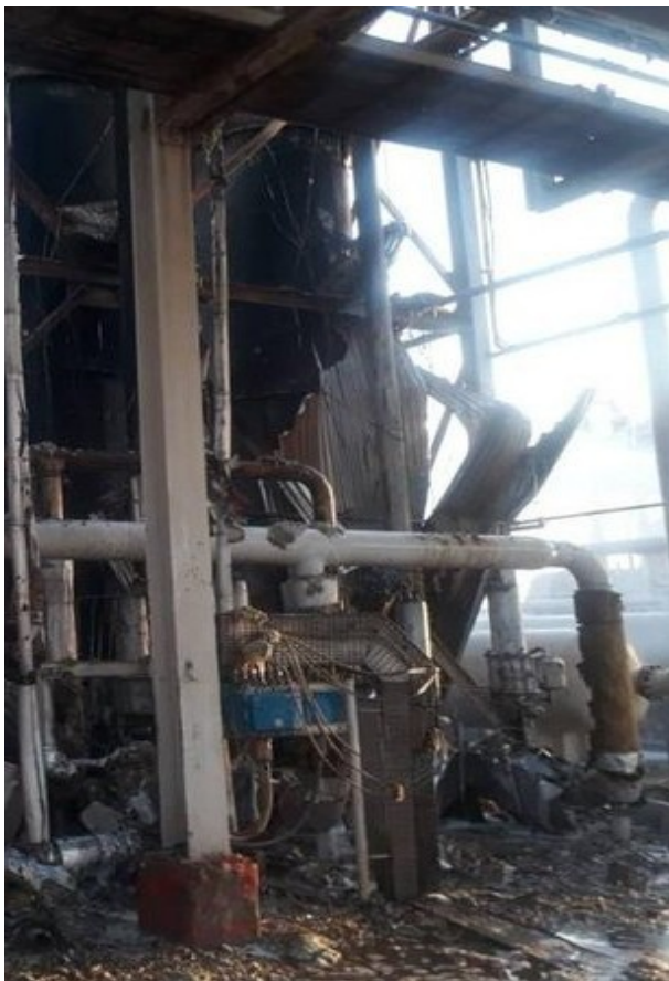
Destroyed gas infrastructure in Suwaidiyah
